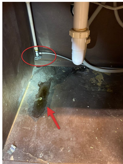
Water shutoff valve to dishwasher was leaking.
