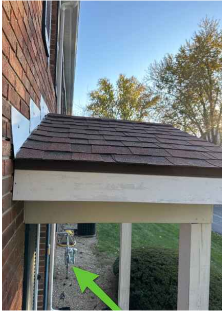
Main gas shut-off valve
